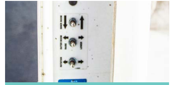
Upper controls including emergency start/stop and variable speed control
